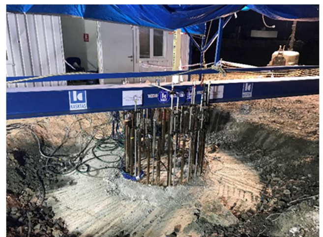
O-Cell® test in progress on the European side. The steel beam is for reference for the measurement of vertical movements
