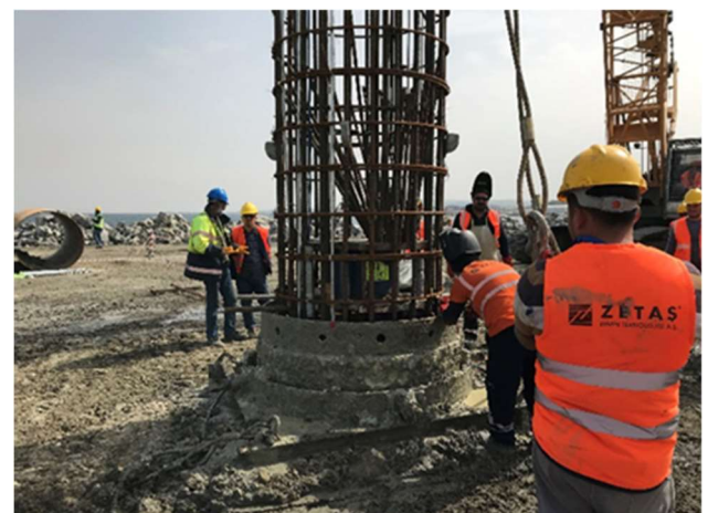
Reinforcing cage, O-Cell® and instrumentation being installed into the pile bore (Asian side)
